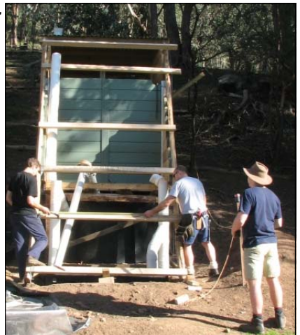
Gareth, Brad and Tom Woods lending their collective skill to the construction of the Rota-Loo.
